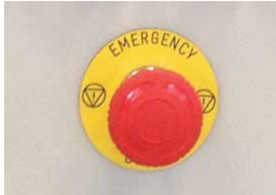
Fig. 2.4 E-stop of the system on main control panel
