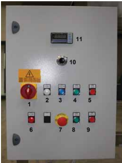
Fig. 5.1 Main control panel
